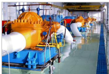
Pump station of the Baltic pipeline system, Transneft
